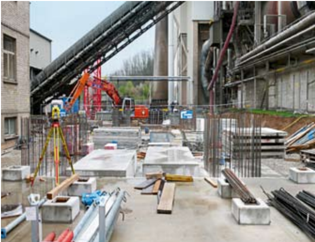
5 Foundation construction work for cooling air fans and pier #3 (left), as well as the completed pier with 3 cooler fans on two levels
