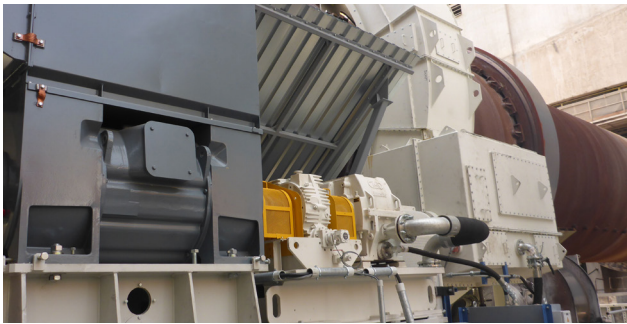
Kiln drive diagnostics
